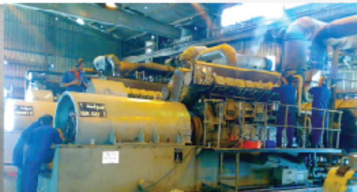
5000 KW - 13.8 KV GENERATOR
