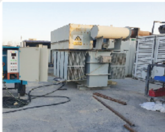
TRANSFORMER OIL FILTRATION MACHINE ON SITE
