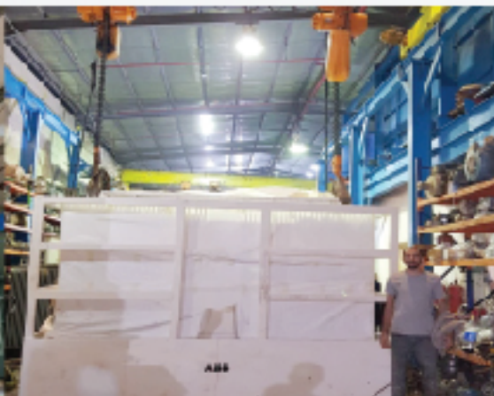
13.8 KV 5000 KVA TRANSFORMER
