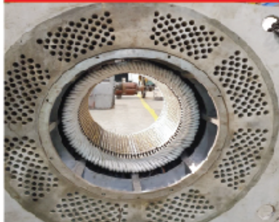
13.8 KV - 3000 HP STATOR REWIND
